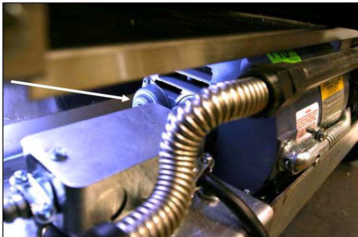
Filter Pump Reset Switch (Arrow)
